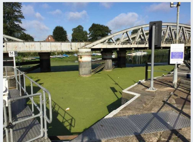
Aquatic weed build up upstream of Grand Sluice.
