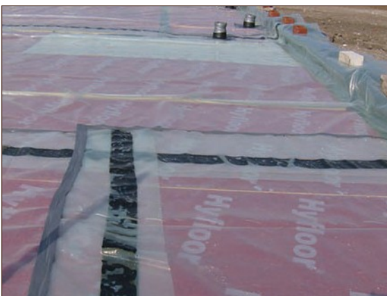
Figure A4.65 Wrinkling of gas membrane over joint has resulted in gaps (only visible due to the use of a transparent gas membrane) and the secondary seal uses ordinary gaffer tape rather than a proprietary product (courtesy Smith Grant)
