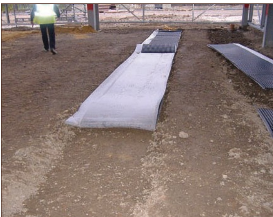
Figure A4.35 Good installation of passive gas venting trenches and 'egg-crate' (courtesy Card Geotechnics Limited)
