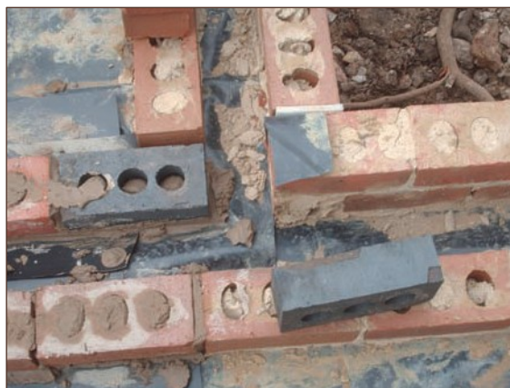
Figure A4.66 Follow-on trades proceeded work before gas membrane joints sealed (courtesy Card Geotechnics Limited)
