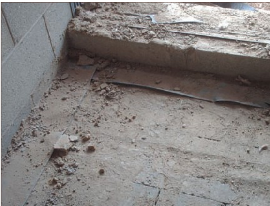
Figure A4.63 Absence of surface preparation prior to laying of gas membrane, debris likely to pierce gas membrane (courtesy Card Geotechnics Limited)
