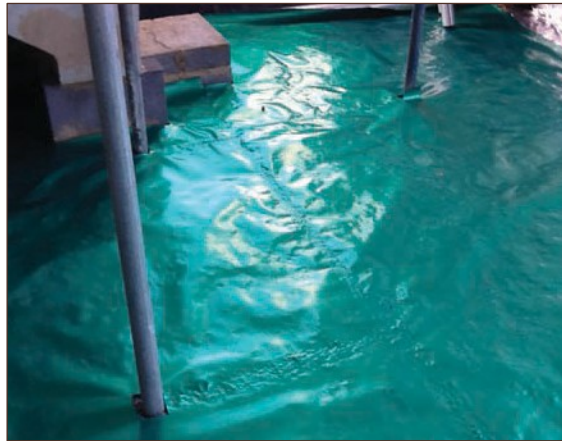
Figure A4.52 Gas membrane cut by scaffolders and bricklayers after installation (courtesy MEC Environmental Ltd)
