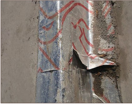
Figure A4.55 Gas membrane at stepped junction of slab to integral garage, appears to be susceptible to tearing when screed is poured. Screed may also weigh down on gas membrane if fitted too tight (courtesy NHBC)
