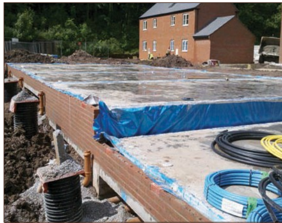
Figure A4.82 Gas membrane used to bridge cavity wall instead of DPC, leaving it exposed to damage by follow-on trades (courtesy Smith Grant)
