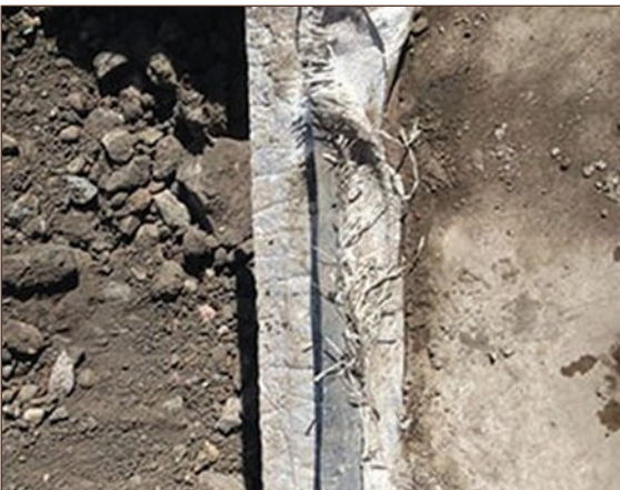
Figure A4.53 Gas membrane left exposed for long period of time, shows significant fraying at cavity edge (courtesy NHBC)
