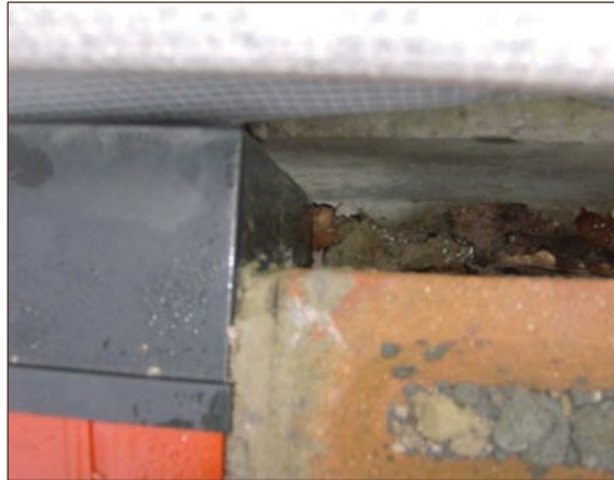
Figure A4.86 Cavity is becoming blocked with detritus. The vent holes in the beam are no longer visible (courtesy Smith Grant)
