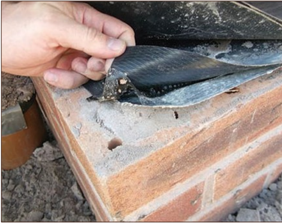
Figure A4.13 Gas proof DPC adhered on top of gas membrane using butyl strips across cavity space (courtesy NHBC)
