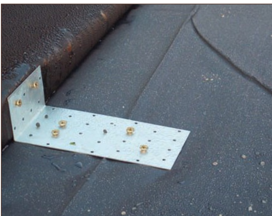
Figure A4.47 Follow-on works purposefully penetrating gas membrane (courtesy Card Geotechnics Limited)
