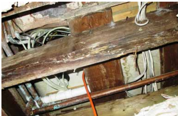
An electric cable through the ceiling from the pub to the en-suite bathroom, to power kitchen equipment located in the bathroom
